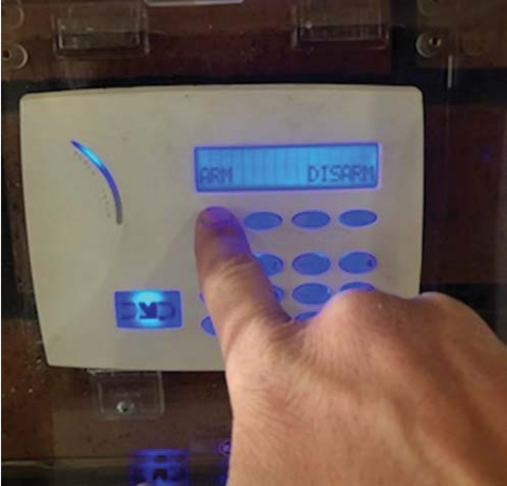
Intrusion Alarm Keypad
