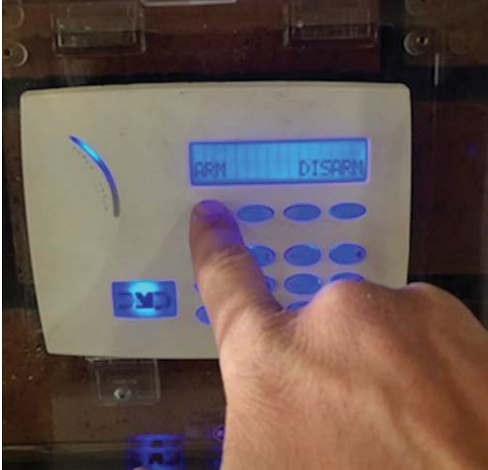
Intrusion Alarm Keypad
